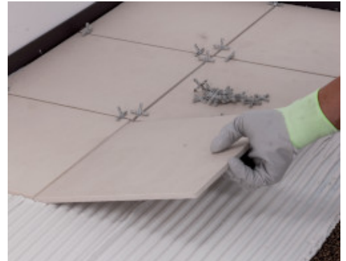
Spread the adhesive on the Mapesonic CR and bond the new floor finish
